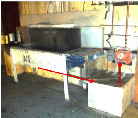
Photo 2: Washtub (Tub02) and above grade tank on east side of the building
