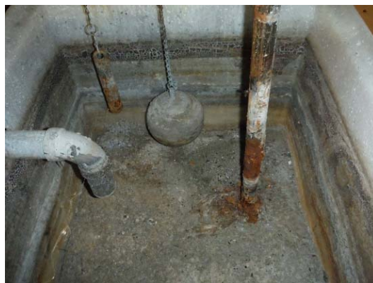
Photo 3: Interior of above grade tank on east side of building, ball float and piping present, associated with Tub02
